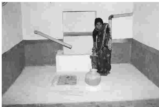
Storage tank inside the house
